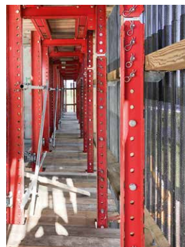
Platforms are protected against the wind during both the construction phase and the climbing phase
