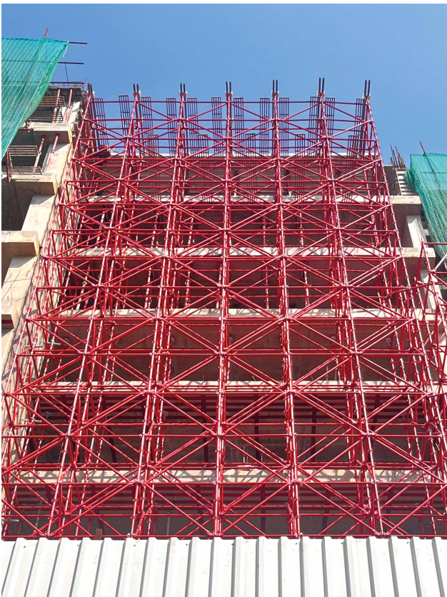
Left: MevaScaff, 34 m high. Next page: Impressions of MonoWal and the project, executed with great skill.
