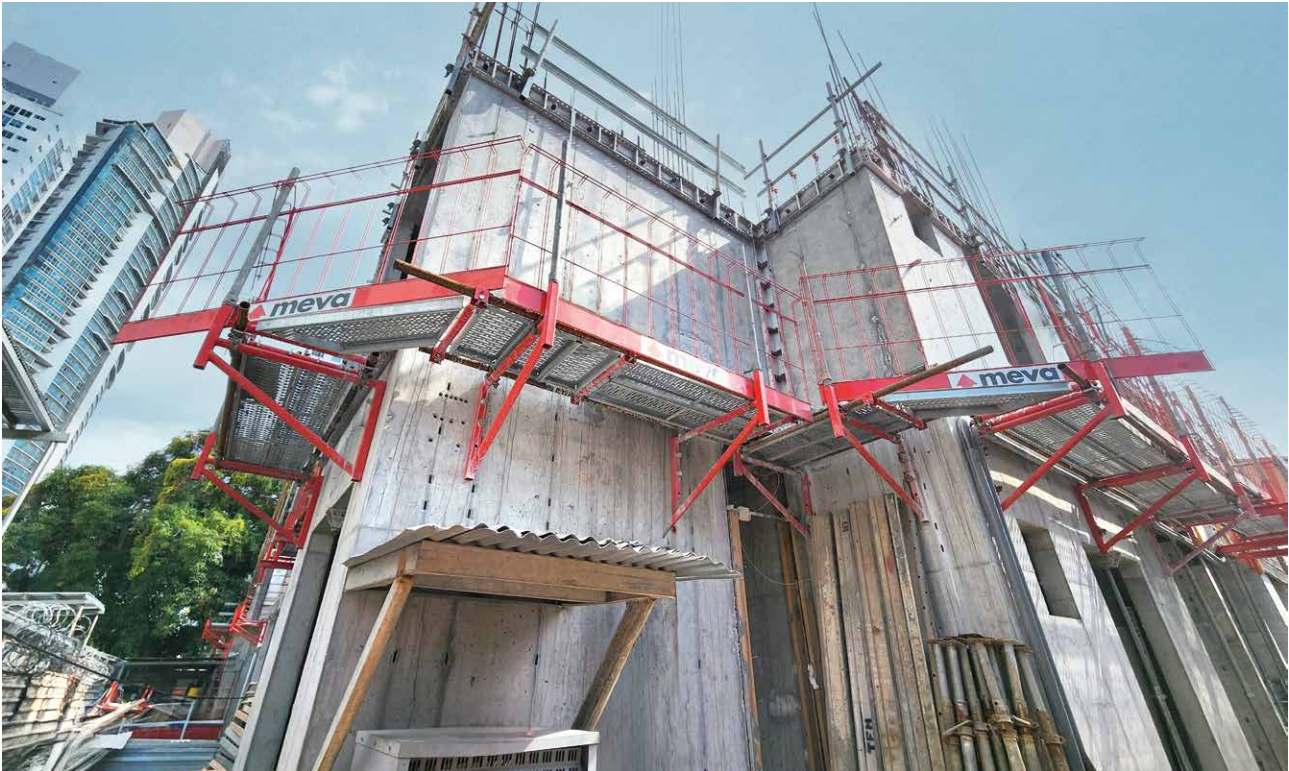
Mono Safety platforms with anti-slip profiling and guard railing allowed the work to be completed safely and comfortably.
