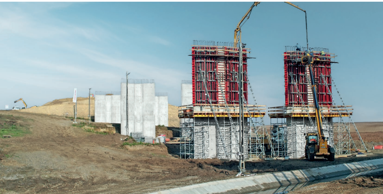
The MT 60 system supports the formwork and the working platforms, and Triplex heavy-duty props transfer the fresh-concrete pressure into the ground.
