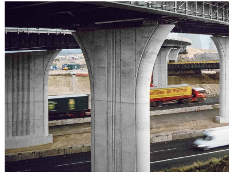
Special formwork can be produced for inclined and curved structures on the basis of the Circo circular column formwork. For example, at the Holmfild Exchange in the UK.
