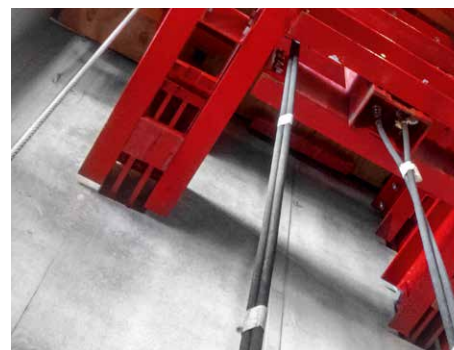
The bearing pockets are removed from the trailing platform and reused during the next climbing stage. This reduces the material costs, as no lost build-in parts are left over in the concrete.
