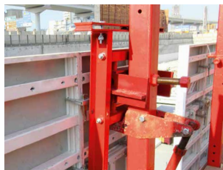
The 3-way adjustment allows for utmost precision. The suspended formwork can be moved and adjusted manually in three directions and can thus be quickly and easily adapted to suit the geometry of the building.
