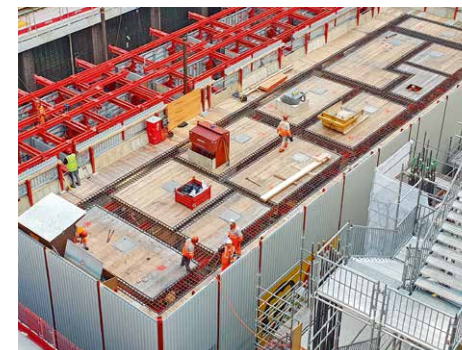
The top deck of the MAC is free of jacking masts, thus ensuring an optimum level of safety, a minimum risk of accidents and more storage space.
