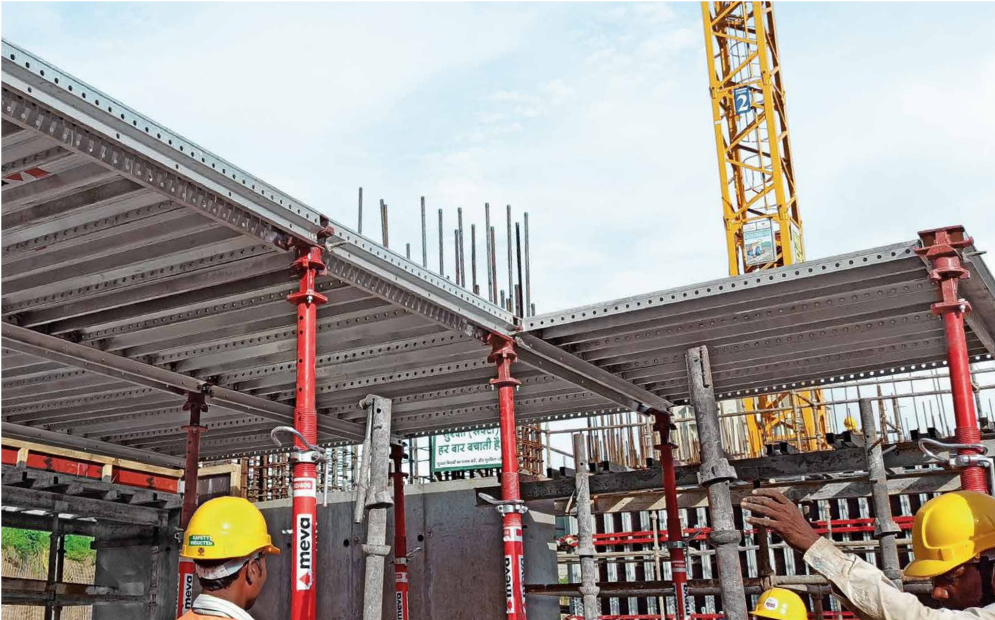
Above and right: The MonoDec slab formwork allows for an early stripping procedure with the use of props with the drop head beams. Below: MSC 240 climbing scaffold and MBS wall formwork – an efficient combination for construction of the lift cores.
