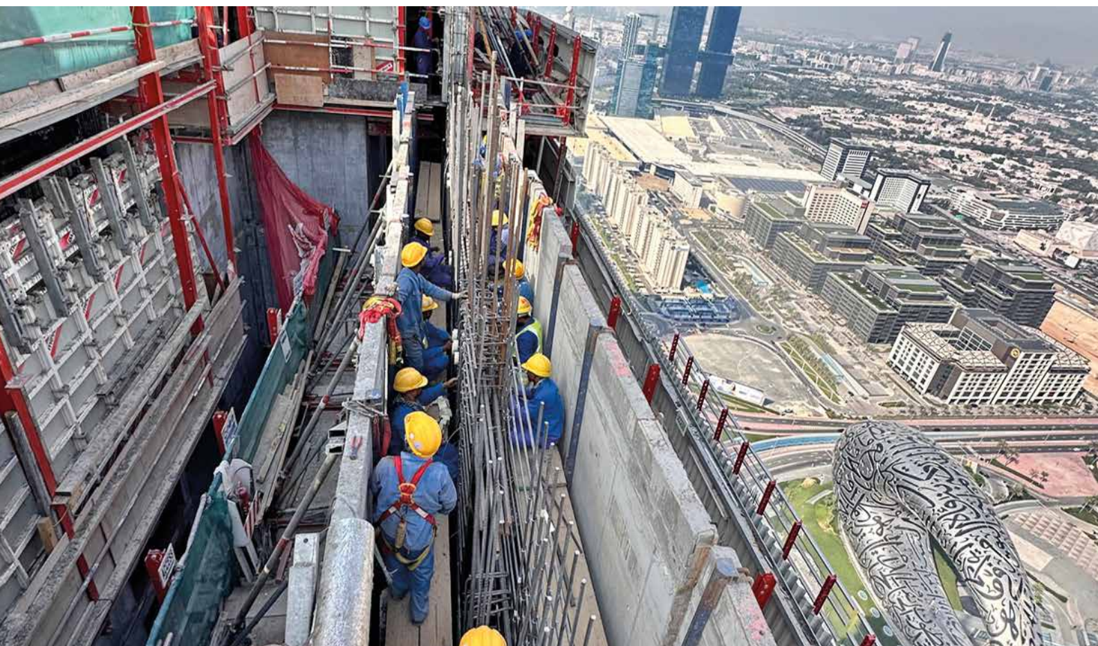
DCC workers and view of Dubai with the Museum of the Future (bottom right). The AluFix formwork can be seen on the left.
